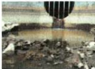
Polluted pool below outfall
