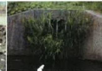
Excessive vegetation below outfall (indicates excessive nutrients in runoff)
