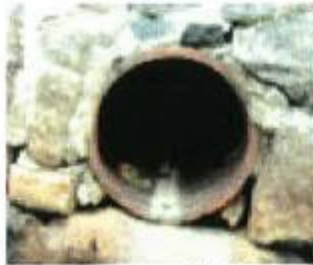
Stains on outfall pipe
